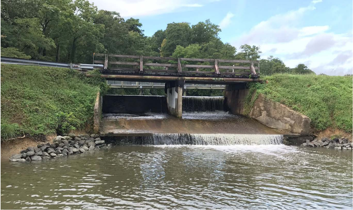
Photo 3 – Existing concrete spillway under the wooden bridge (bare slopes on both sides)
