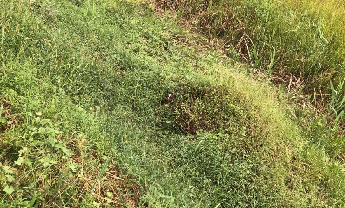
Photo 5 – Buried Stump near downstream toe of dam (rotting wood is forming holes)
