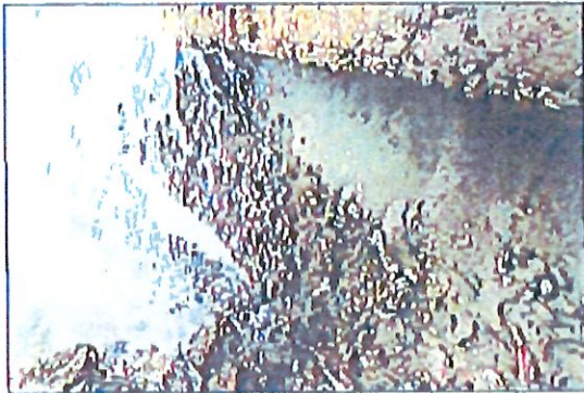
01.19: CONCRETE BELOW THE WATER LINE IS COVERED WITH BARNACLES
