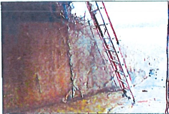
01.10: THERE IS A COLD JOINT BETWEEN THE WINGWALL AND THE ABUTMENT, AND ALSO AT THE BASE OF THE WINGWALL
