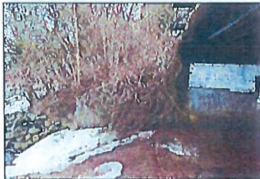
01.14: SPILLWAY CRACK LOOKING TOWARDS THE EAST ABUTMENT
