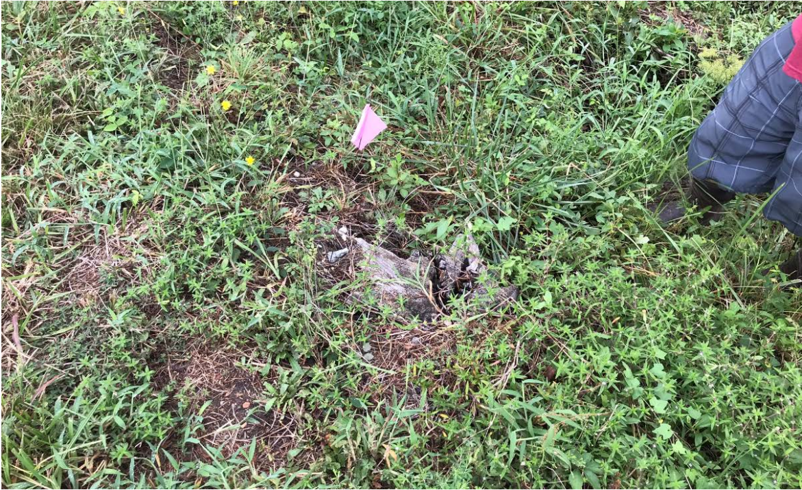
Photo 6 – Buried Stump near downstream toe of dam (pink flags note holes forming)
