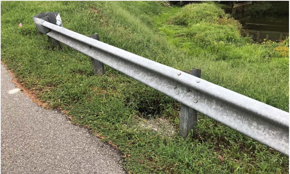
Photo 2 – Holes under the Guard Rail Posts (being addressed by VDOT)
