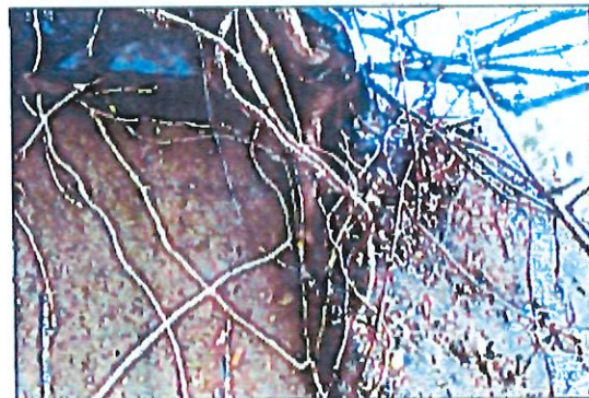
01.11: LARGE ROOTS ARE FORCING THE COLD JOINT TO SEPARATE
