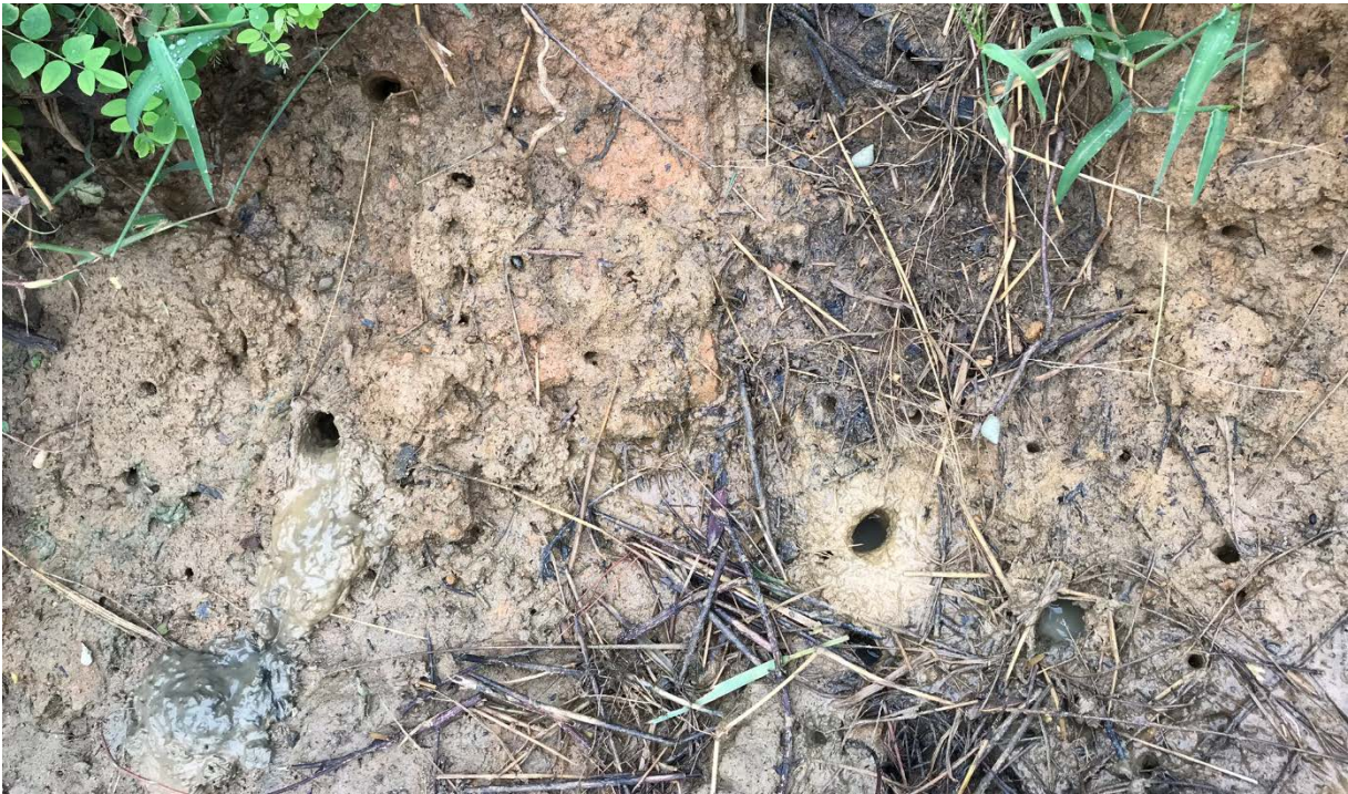
Photo 4 – Small crabs and holes in the embankment near the concrete spillway
