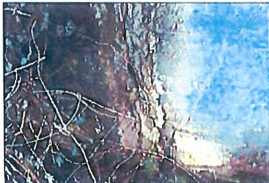
01.16: CRACK AND SPALL IN THE EAST ABUTMENT AT WING WALL
