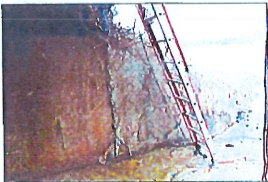
01.10: THERE IS A COLD JOINT BETWEEN THE WINGWALL AND THE ABUTMENT, AND ALSO AT THE BASE OF THE WINGWALL
