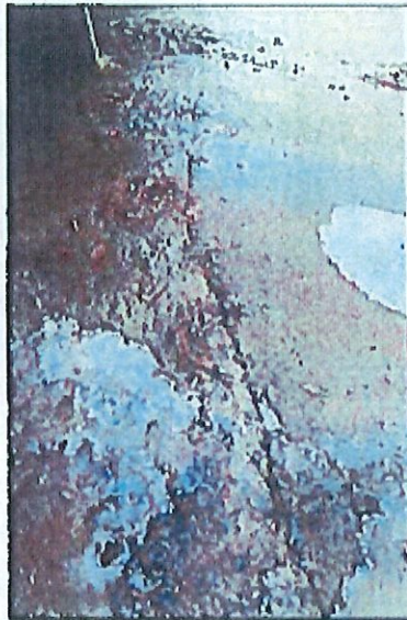
01.12: CRACK ACROSS SPILLWAY
