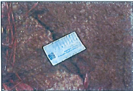
01.13: SPILLWAY CRACK VARIES FROM ABOUT 1/4" TO HAIRLINE
